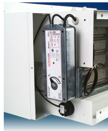
Figure 1. Image showing the side access cover removed exposing the motor cassette and ETR probe.
